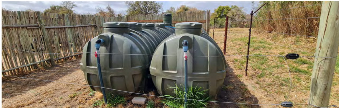
Wastewater treatment plant at Imbali Safari Lodge
