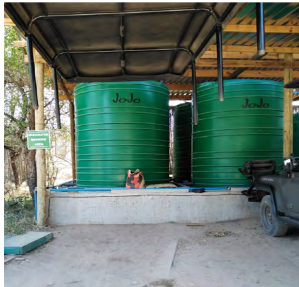
Grey water reticulation installed, and grey water used for car wash, watering of gardens etc.
