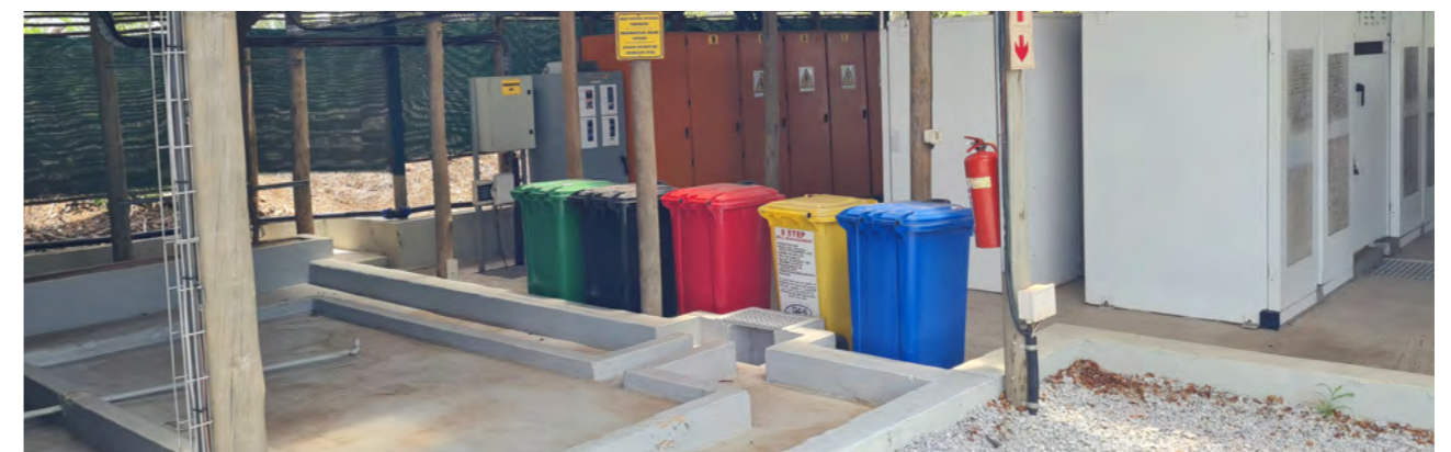
Fuel storage area bunded at Singita Lebombo.
