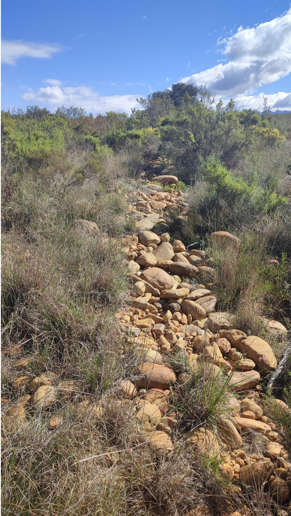
Photo 9: Section through veld where new soakaway pipelines will be laid along existing soakaway pipeline to the new soakaway. (Photo taken 17/08/2022).
