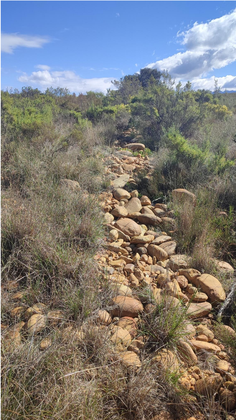
Photo 7: Section through veld where new soakaway pipelines will be laid along existing soakaway pipeline to the new soakaway. (Photo taken 17/08/2022).
