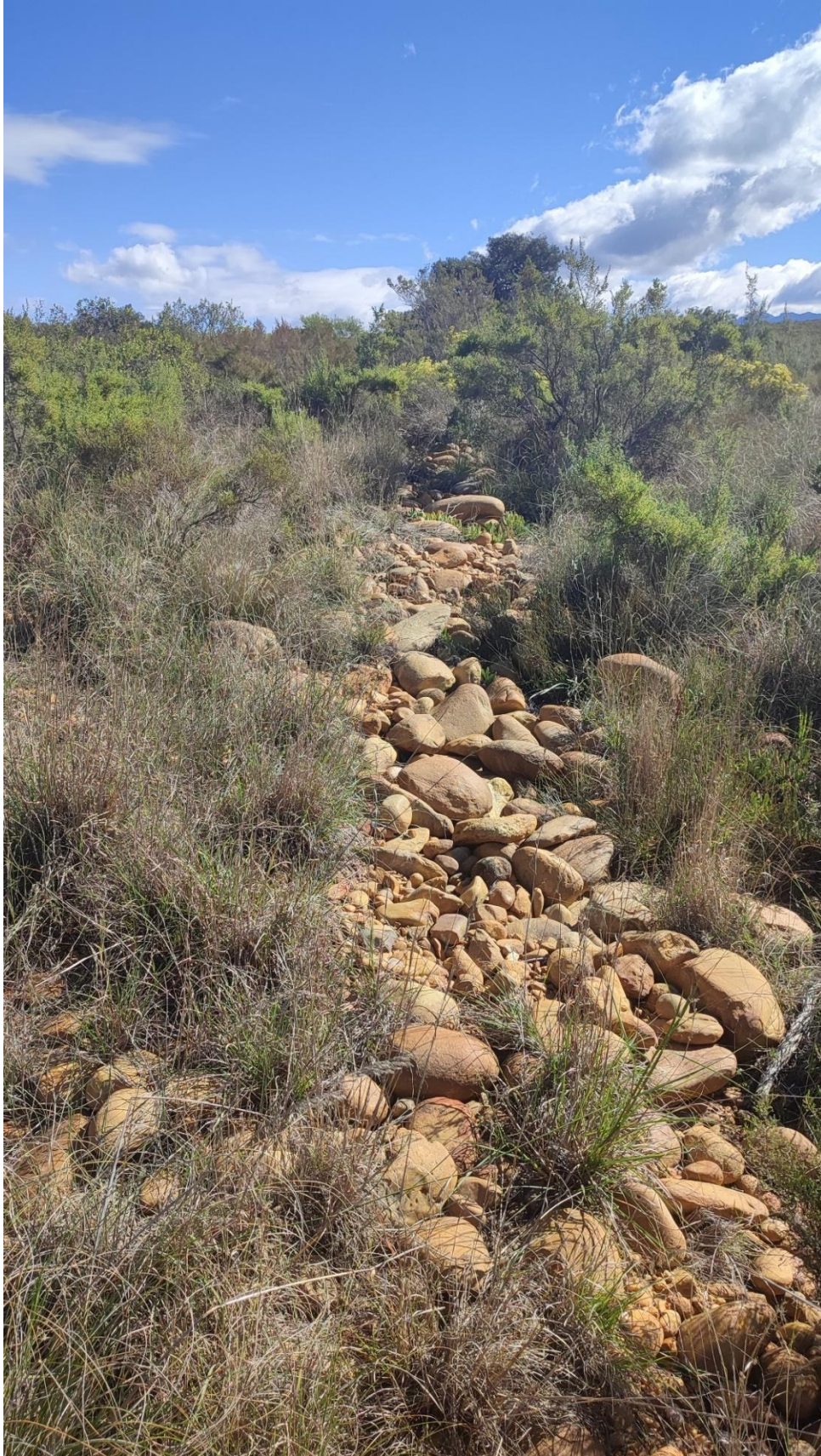
Photo 7: Section through veld where new soakaway pipelines will be laid along existing soakaway pipeline to the new soakaway. (Photo taken 17/08/2022).
