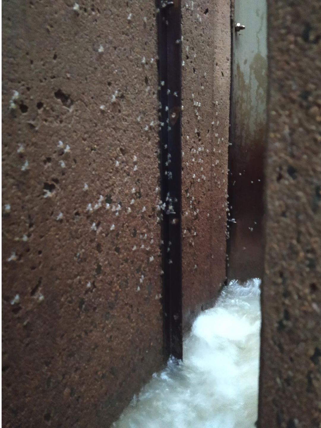
↓ Second baffle in the fishway
