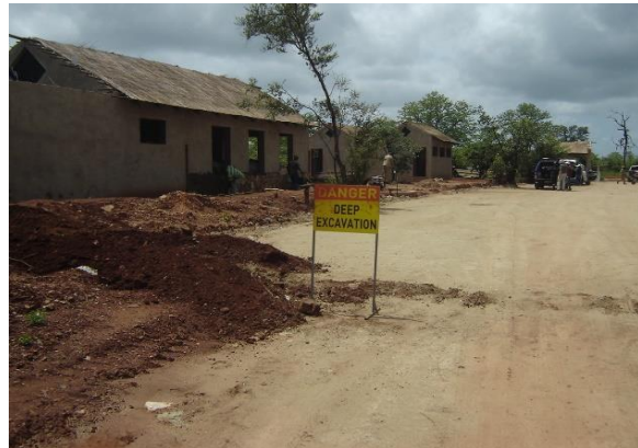
Danger tape is erected on site.
