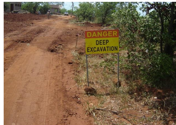
Danger tape is erected on site.
