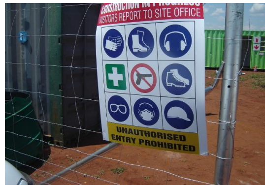
There is a fire extinguisher on site.
