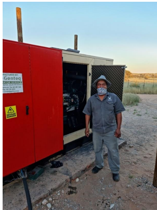
Figure 14: Mata Mata Generator Location
