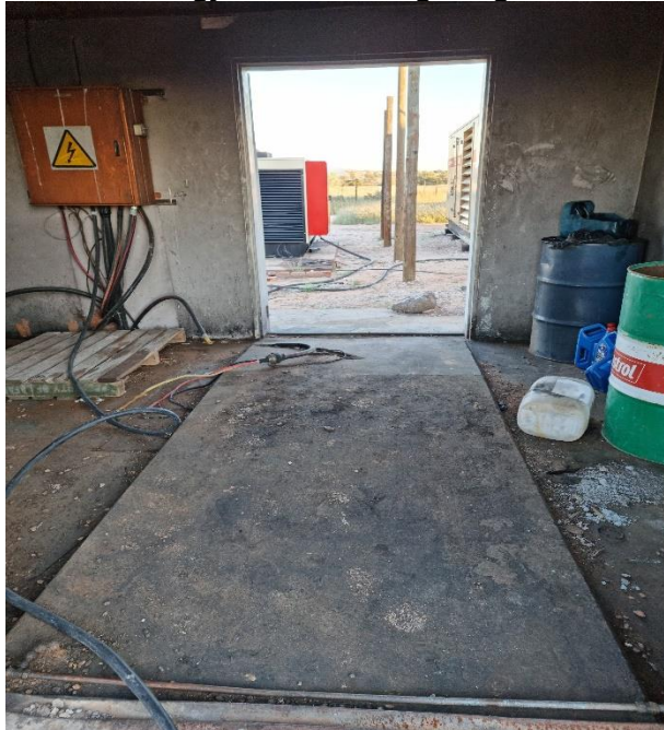
Figure 17: Mata Mata Energy Room with Generator
