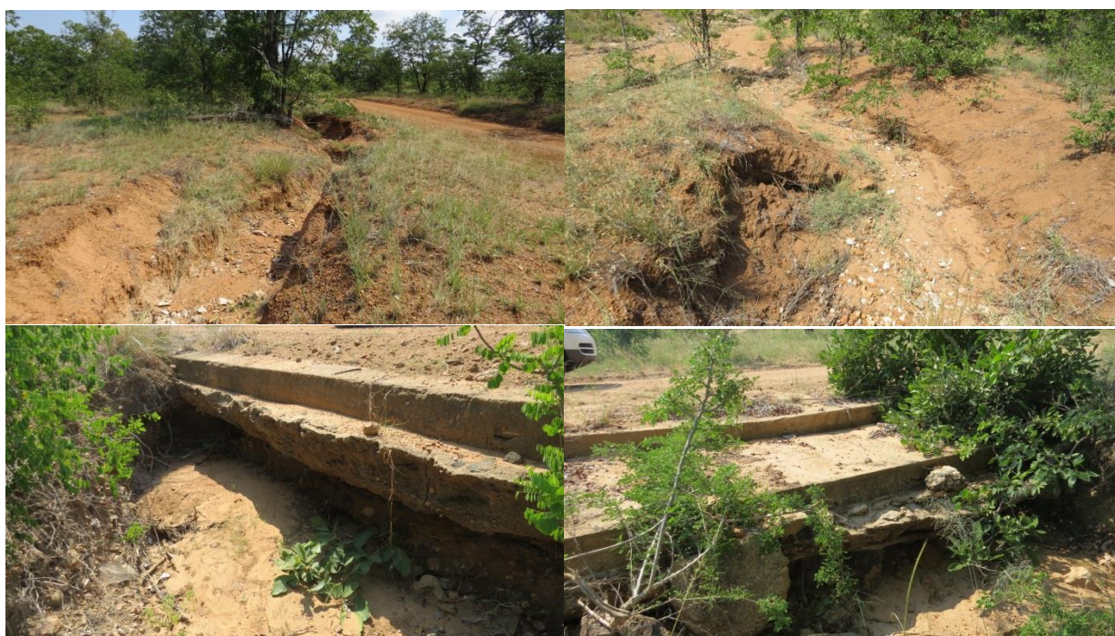
Figure 16: Figures indicating erosion associated with the rivers and the low water bridges.
