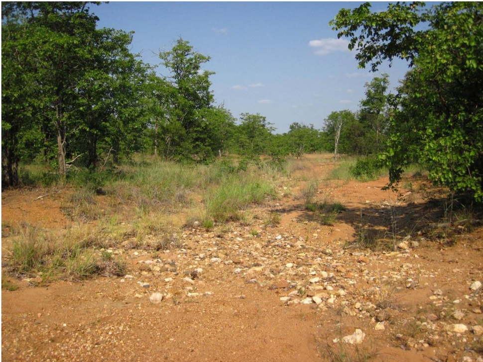
Figure 17: One of many storm water drainage lines along the Shangoni Ranger patrol road at 23° 10' 08.8"S; 31° 06' 41.5"E.
