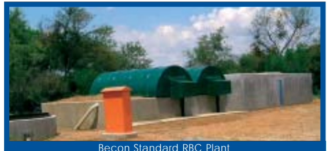
Becon Standard RBC Plant
