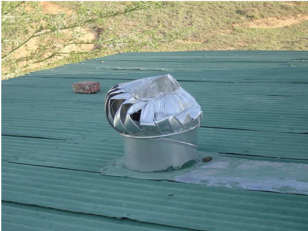
Figure 12: River Lodge dilapidation
