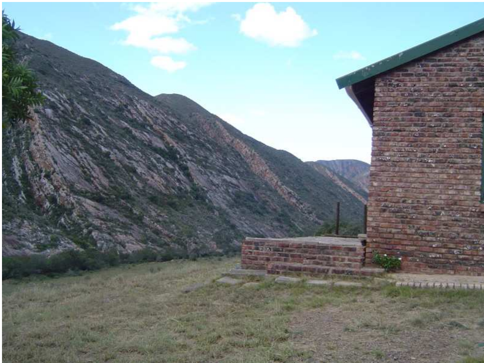
Figure 10: Prospect House (requires refurbishing)
